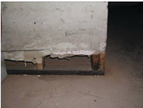
Figure 1-11 Gypsum board on the lower edge of a basement wall dissolved by seasonal flood waters. The water table is just below the basement floor during dry weather and rises several inches above the floor during heavy spring rains.
