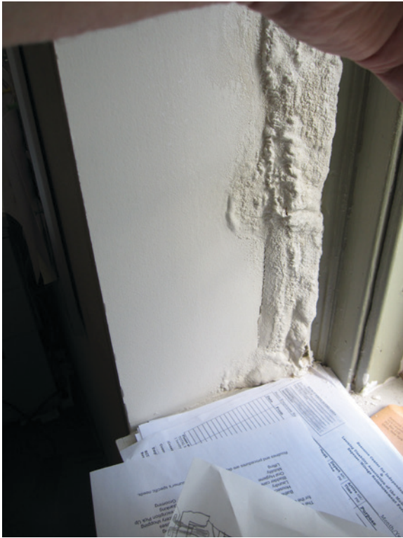
Figure 1-10 Further rain damage to interior plaster. At another location on an office window in the building shown in Figure 1-8, rain seepage turns gypsum board joint compound to a fluid, causing the gypsum to bubble and lift.
