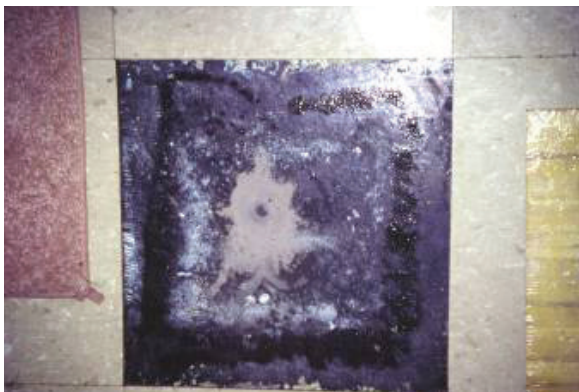
Figure 1-13 Tile adhesive that failed to cure because of water in the concrete and high pH. The tile can be removed by hand. The floor is a concrete slab-on-grade. The water visible in the photo evaporates into the room after several minutes. Its source may be liquid water wicking up from the sub-slab fill or water vapor migrating through the slab.
