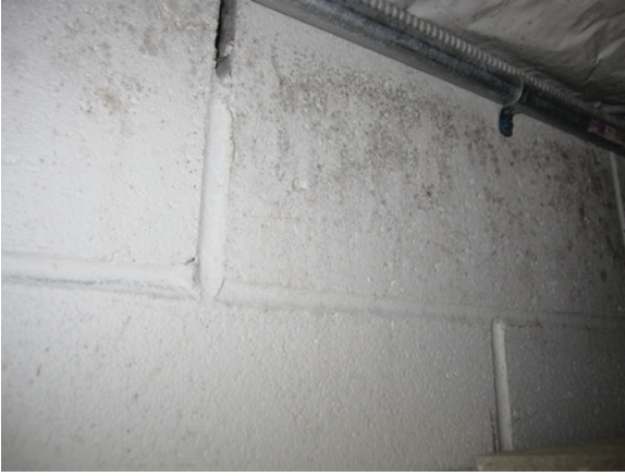
Figure 1-2 Mold growth on painted concrete masonry. The cool masonry wall separates a classroom from an ice rink. Humid air in the classroom provides moisture that condenses on the painted surface of the masonry. That moisture allows mold to grow on the paint film.
