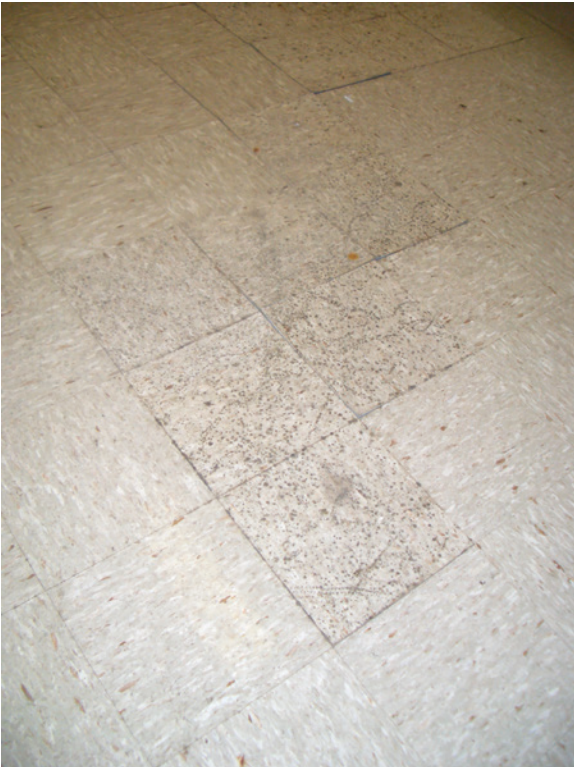
Figure 1-3 Mold growth on vinyl floor tile. Long-term high humidity provided moisture that was absorbed into the cool vinyl tile and supported mold growth. Also note that the high humidity caused the adhesive attaching the tile to the floor to fail, allowing the tile to become loose.
