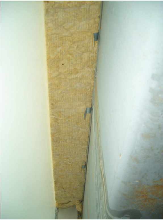
Figure 1-5 Corrosion of structural steel in a ceiling cavity in a cold climate. The steel extends into the exterior wall assembly. During cold weather, the steel near the wall is chilled by cold outdoor air. The building is humidified, and condensation from high indoor humidity provides the moisture that rusts the cold steel.
