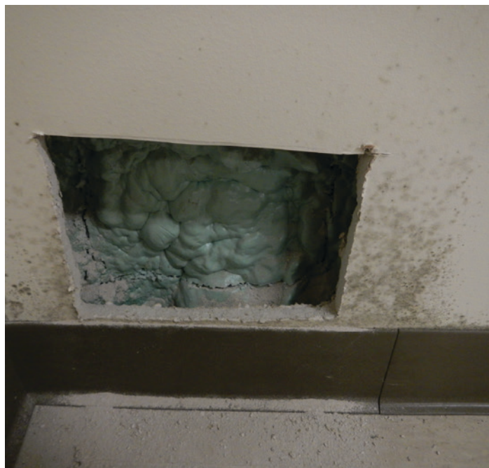
Figure 4-1 Interior Wall Showing Water Damage and Mold
