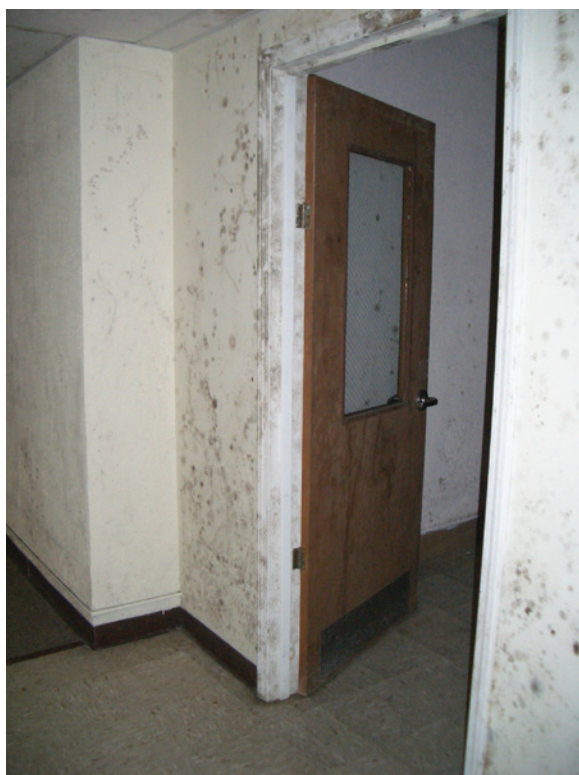
Figure 1-1 Mold growing on the surface of painted gypsum board and trim. Long-term high humidity is the source of the moisture that allowed the mold growth. All of the walls experienced similar near-condensation conditions. Consequently, the mold growth is widespread rather than concentrated in a single damp area.
