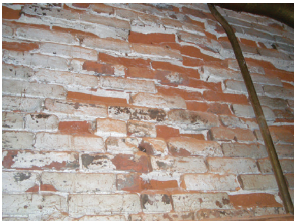
Figure 1-14 Damage to bricks caused by the migration of soluble salt through them. Salts in the brick or mortar dissolve in rainwater that wicks through the brick. The water evaporates in the building's interior, and the salt left behind crystalizes and splits the surface layer off the brick, exposing its interior. This process is called sub-fluorescence.
