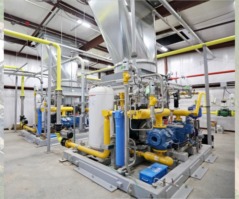
Compressor at Dane County's new RNG offloading station. Photo: Amber Arnold, State Journal
