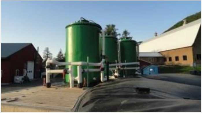
Photo of the three tanks, located adjacent to the digester, that are used to store the feedstock. Photo Credit: Barstow's Longview Farm .
