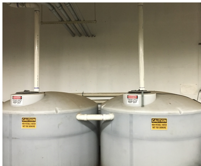
Storage tanks for rainwater collected from roof drains.
