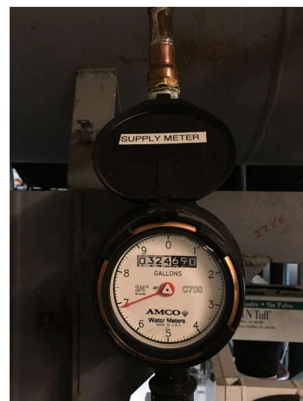
Cooling tower make-up meter.
