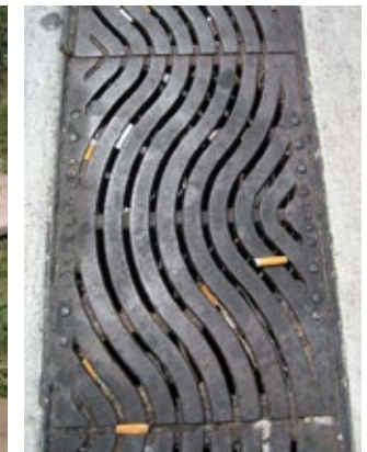
Figure 4-28. The small spaces in this grate are clogged with cigarette butts, which block drainage and are difficult to remove.
