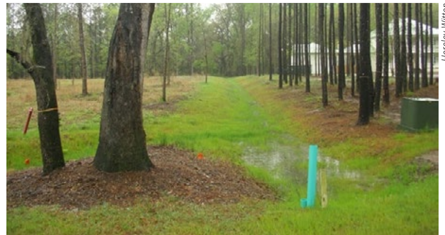
Infiltration trench with grass cover.
