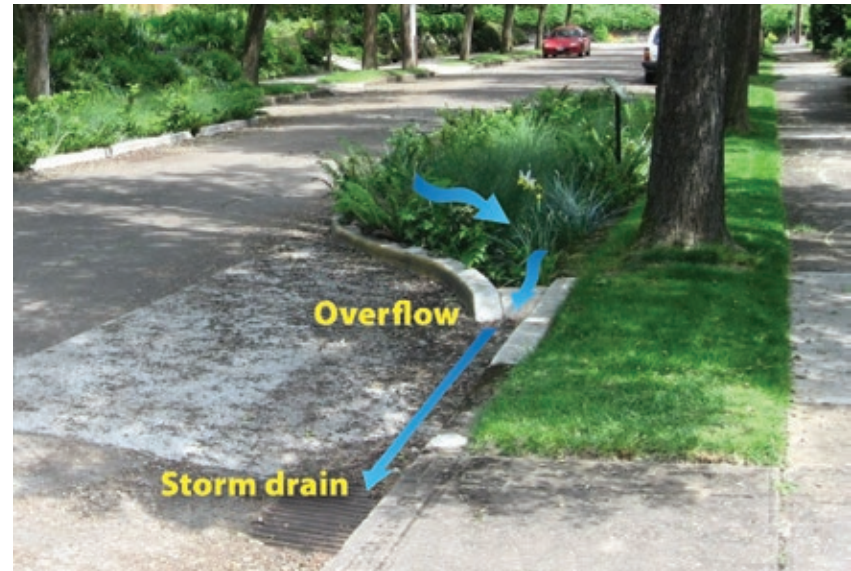
Runoff enters the upper end of this curb extension, and the overflow volume exits through an opening on the lower end and drops into a storm drain.
