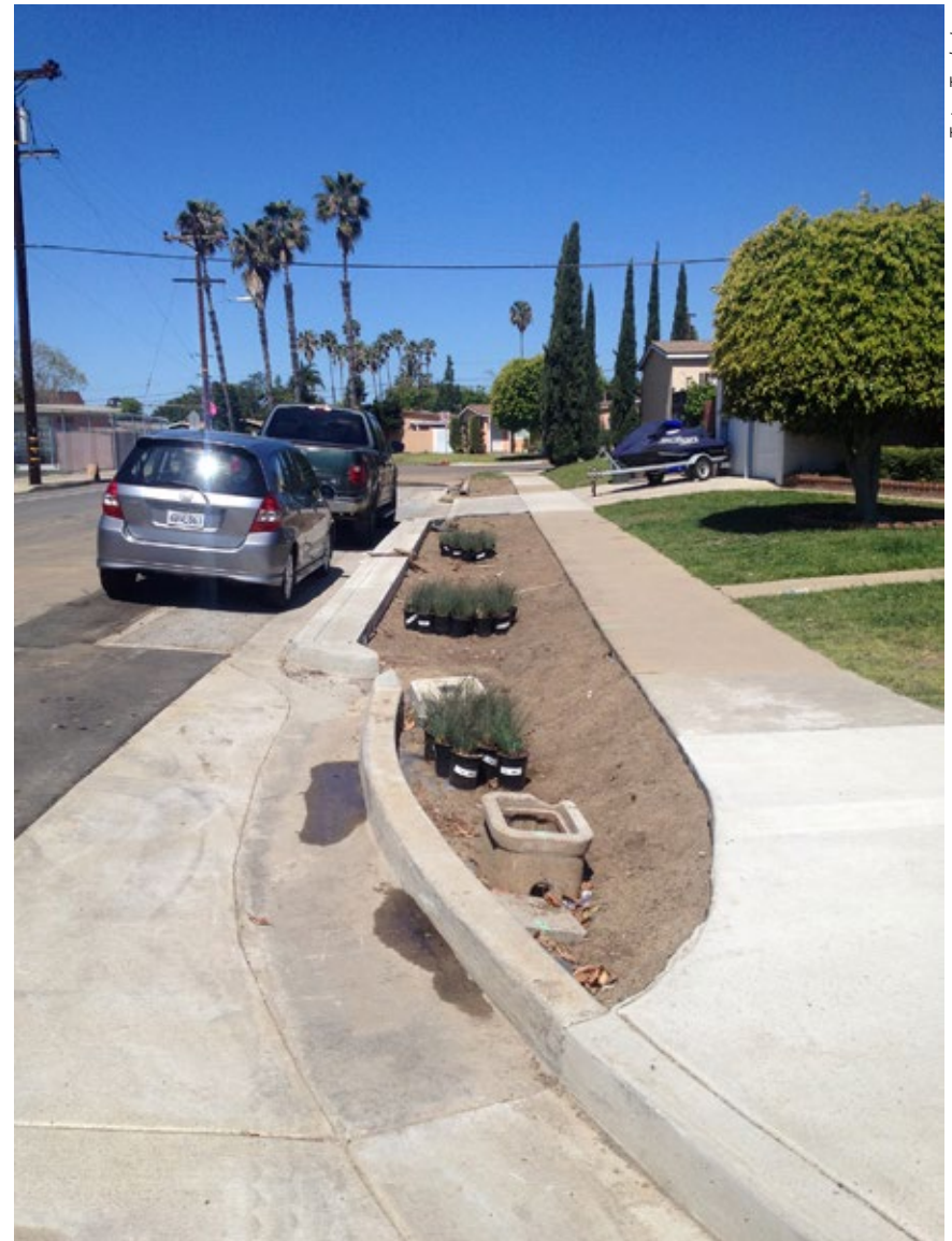
In preparation for planting local native vegetation, a soil media mix was chosen and backfilled into this roadside bioretention area in San Diego, CA.
