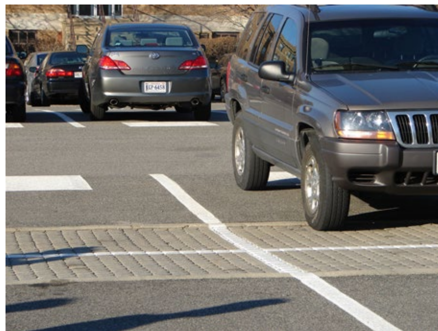
Permeable pavers installed at the downgradient end of parking bays collect surface runoff and allow it to infiltrate.
