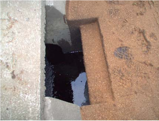
Fig. 7 – Rainwater sewer inlet.
