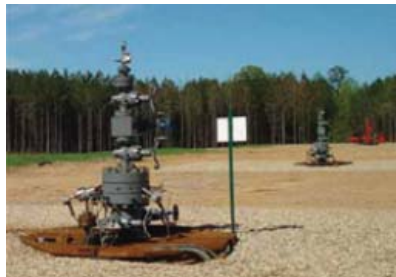
CO 2 Geosequestration Wells Photo courtesy of the U.S. Department of Energy
