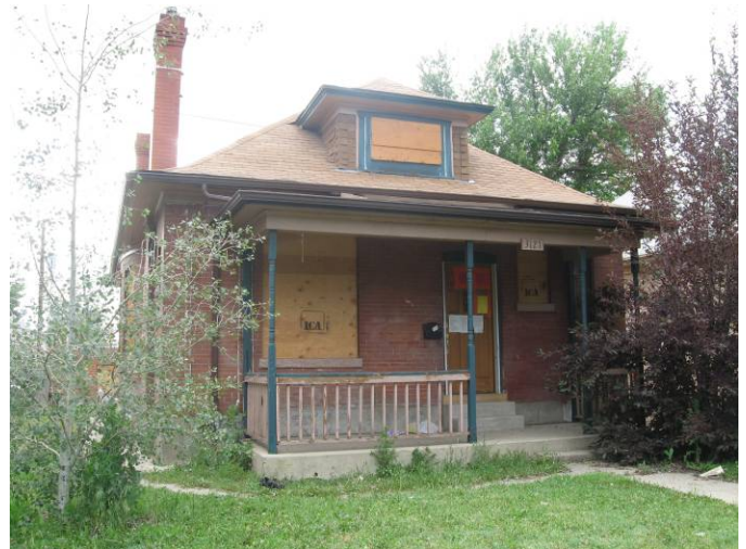
Boarded Up Methamphetamine Laboratories like this one in the Cole neighborhoods were included in GWD's inventory of potential brownfield sites.
