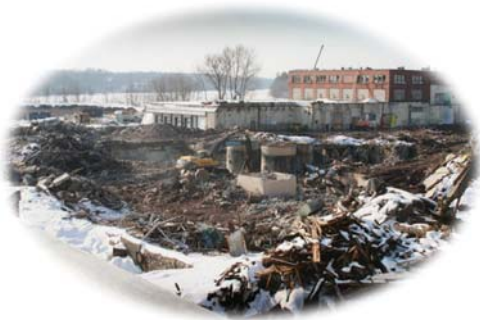
Demolition in progress on main mill buildings at the former Eastern Fine Paper property.
