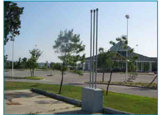
Vent pipes from the UST prior to removal at Swifty Serve gas station in Moss Point, Mississippi.
