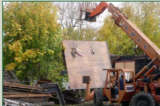
City of Cleveland deconstructing an abandoned building as part of its Deconstruction Initiative program.
