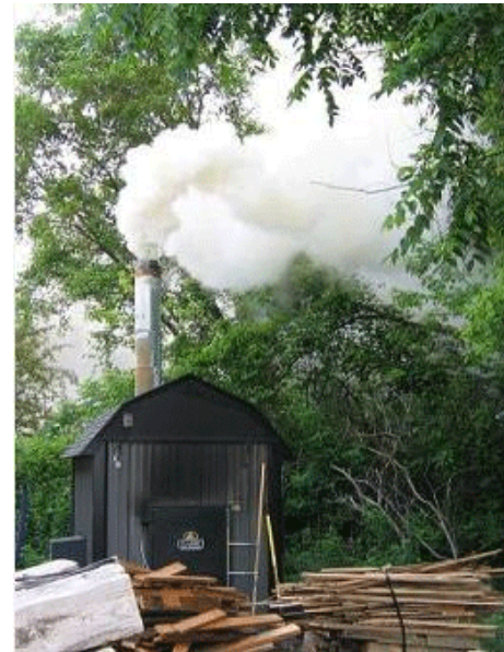
Outdoor Wood Boiler
