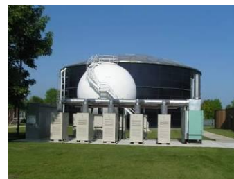
Waste Water Plants
