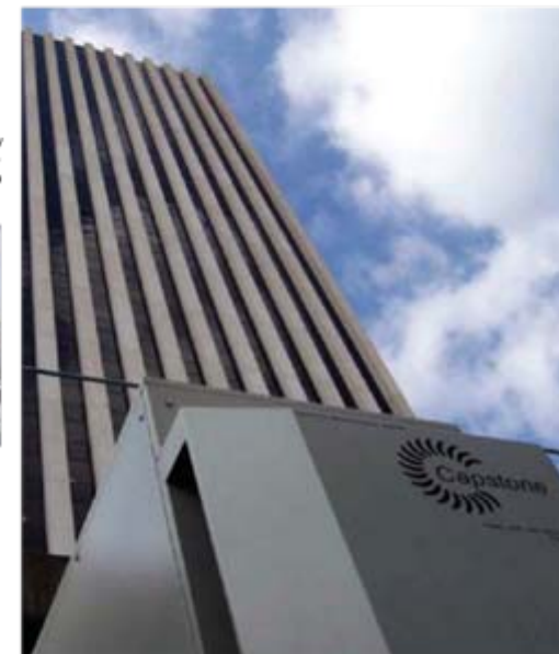
Six Capstone C60 microturbines assure power security at this downtown Houston site.
