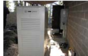
Four C65 Micro Turbines™ running on natural gas provide CCHP at a data center in California.
