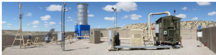
The Solvay Mine methane capture and utilization site Photo courtesy of: Sindicatum
