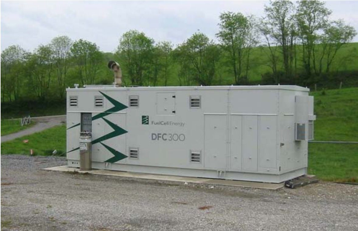
200 kW solid oxide fuel cell (SOFC) sited at AEP Ohio Coal LLC's Rose Valley Mine Site in Hopedale, Ohio.
