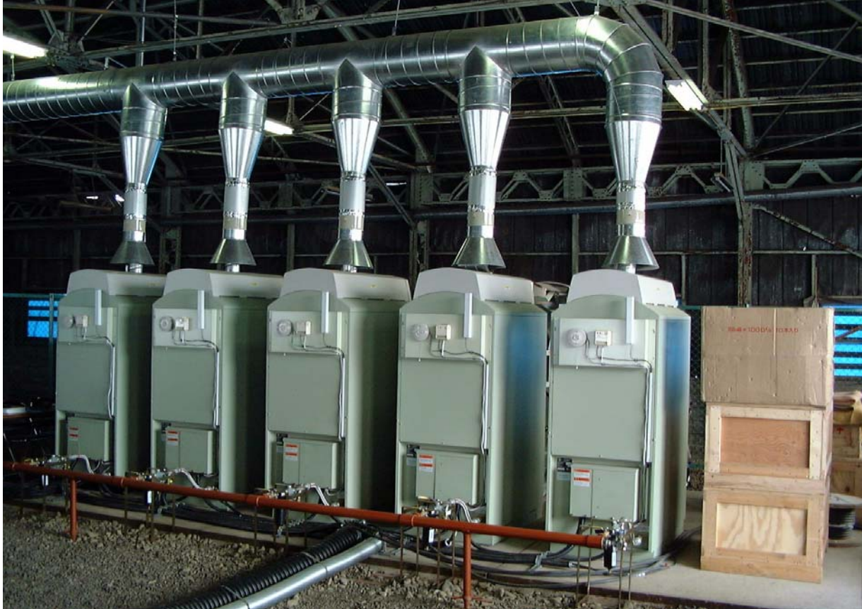
Five Capstones Micro Turbines Operating at abandoned Akabira Mine in Japan (Photo courtesy of Raven Ridge Resources)
