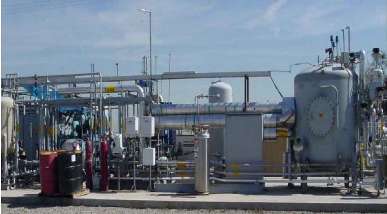
Example of a small scale LNG plant (built by a predecessor company to Prometheus Energy)
