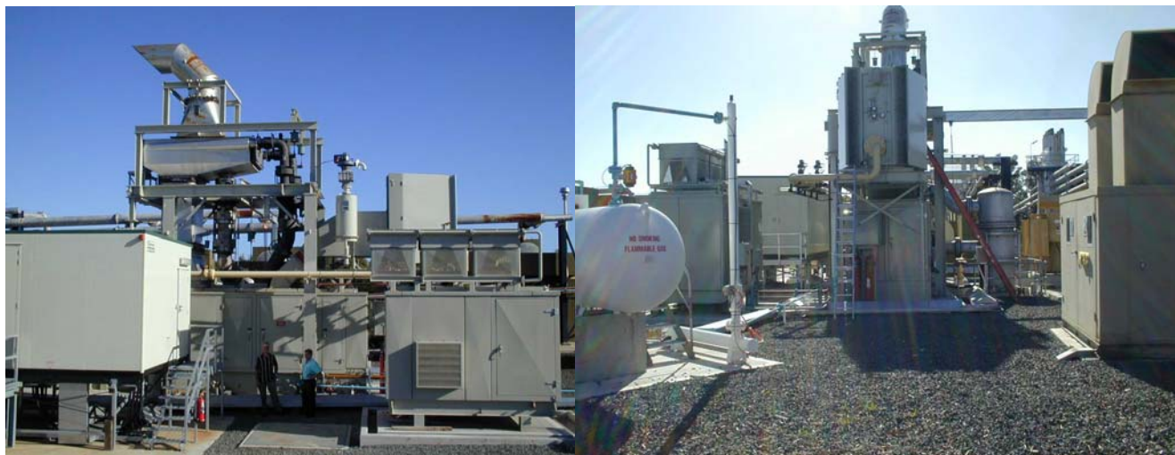
Appin Turbine Installation - Side View & End View, Respectively (Photo courtesy of DUT Pty Ltd)
