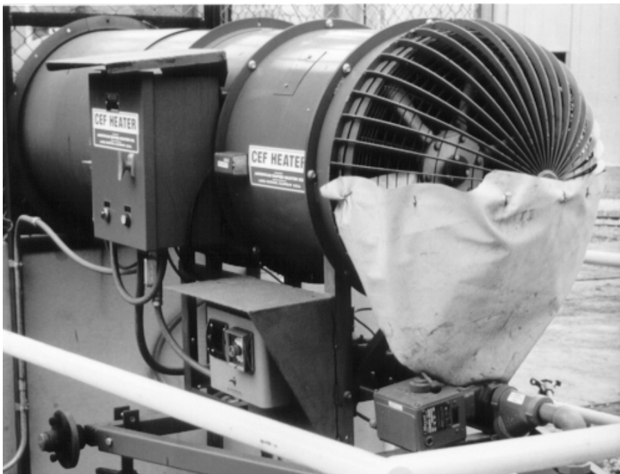
Coal mine methane-fueled heater at one of the Jim Walter Resources mines in Alabama (Photo courtesy of Jim Walter Resources, Inc.)
