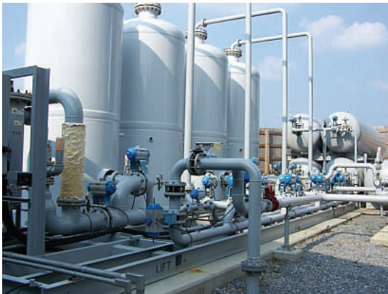
Cambria 33 Gas Plant
