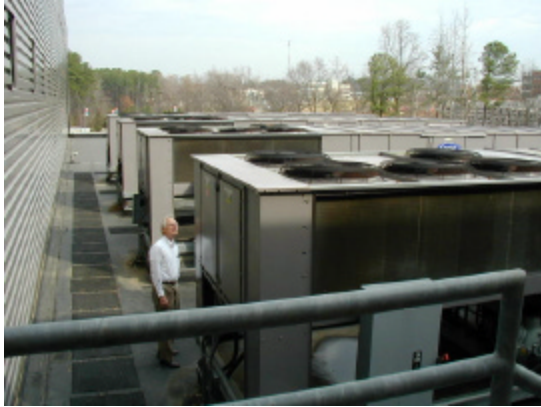
Commercial Roof-Top Air-Conditioning System
