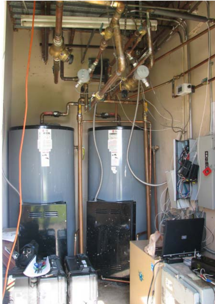
Figure 1-3. Lake Towers Installation
