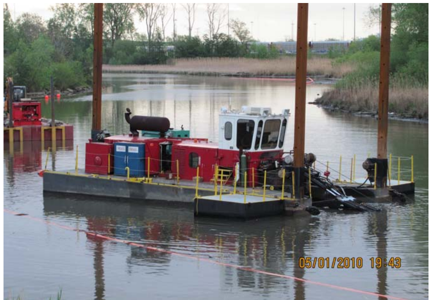
Hydraulic dredging of the Ottawa River is under way in Toledo. The barge shown here holds the booster pumps to help move the sediment to the Hoffman Road Landfill.
