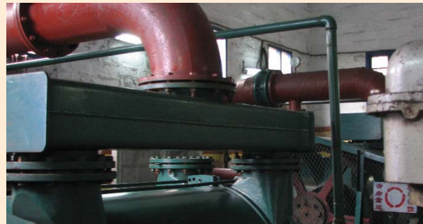
Pumping station at a mine under study in China. The station extracts methane from the underground coal seam in advance of and during mining.
