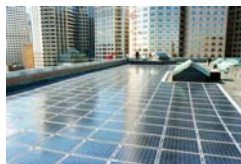
Williams Building, 28 kW (NREL PIX 08466)
