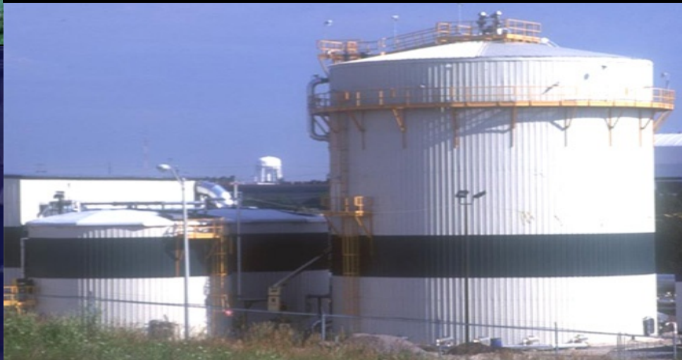
Solid Waste Digester
