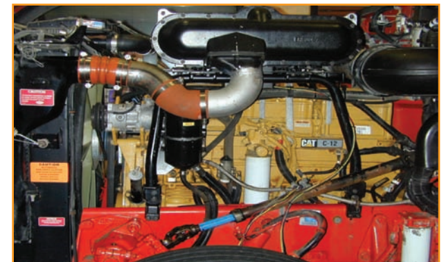
Membranes within the black housing mounted over the diesel engine pictured above generate NEA from cooled turbocharged air.
