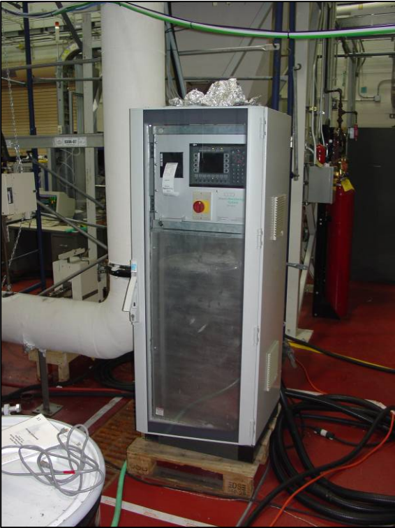
Figure 3-4. DioxinMonitoringSystem Control Unit
