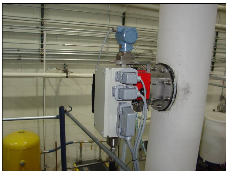
Figure 3-3. Installed DioxinMonitoringSystem Sampling Probe
