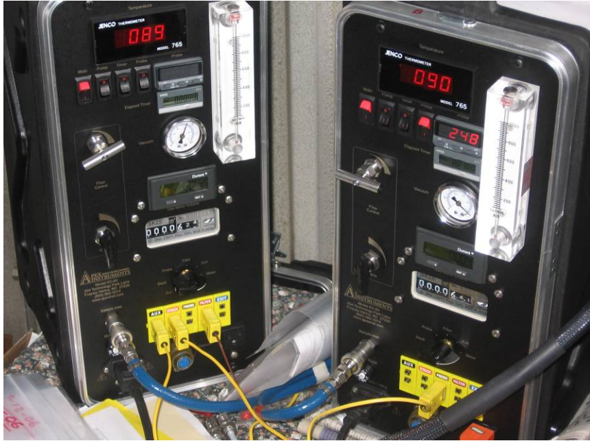
Figure 2-1. Apex XC-60 Gas Sampling Consoles
