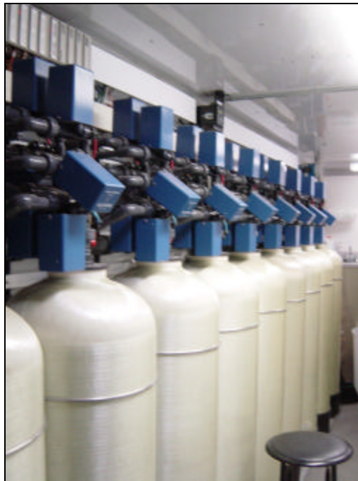
Photograph 2: Interior of Basin Water high efficiency ion exchange system.
