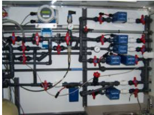
Photograph 6: Brine flow control system.
