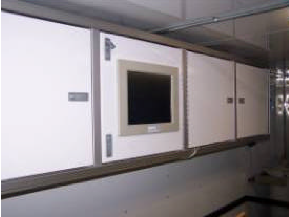
Photograph 4: Data computer and control system.
