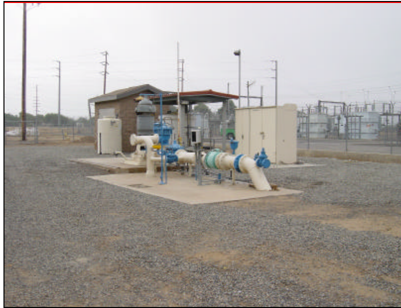
Photograph 1: Test site at the Corydon Street Well.
