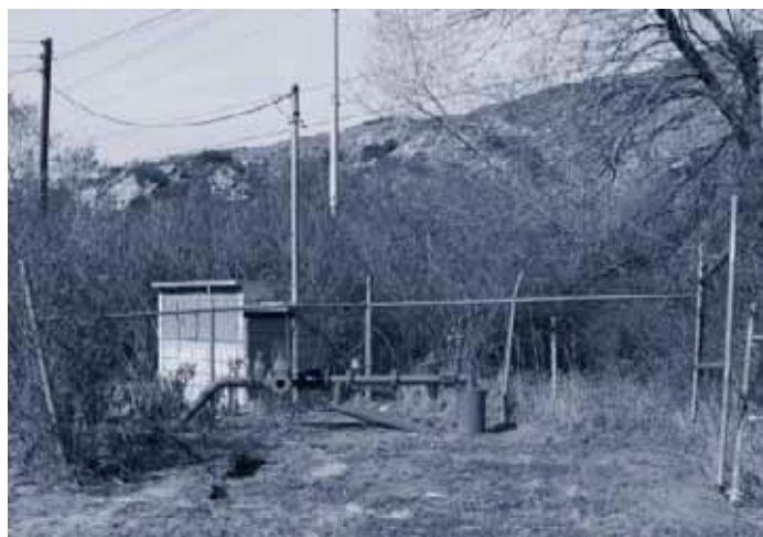
The Tecate Aquifer, being tapped via this well, provides about 15% of the potable water for the city.
