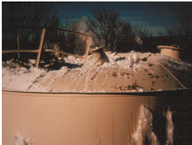
Tank Damaged by Vacuum in Combination with Snow Load
