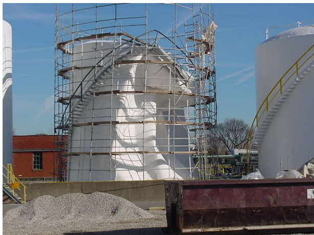
Tank Damaged Beyond Repair by Vacuum
