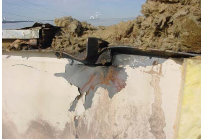
Tank Roof to Shell Connection Damaged by Vacuum
