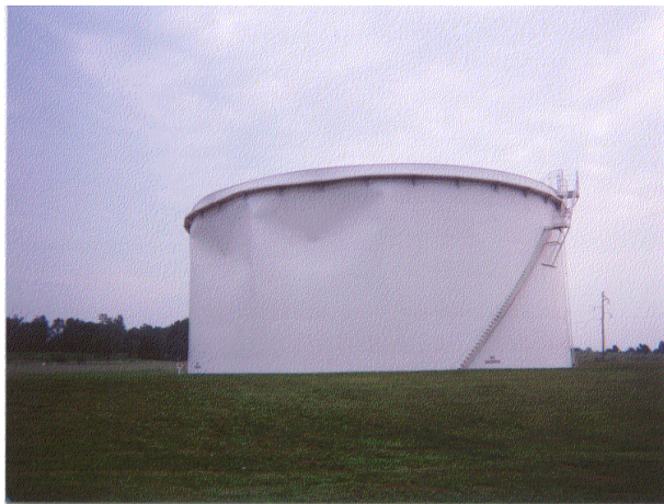
Tank Damaged by Tornado Winds
