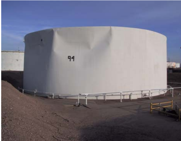
Tank Damaged by Negative Internal Pressure (Vacuum)
