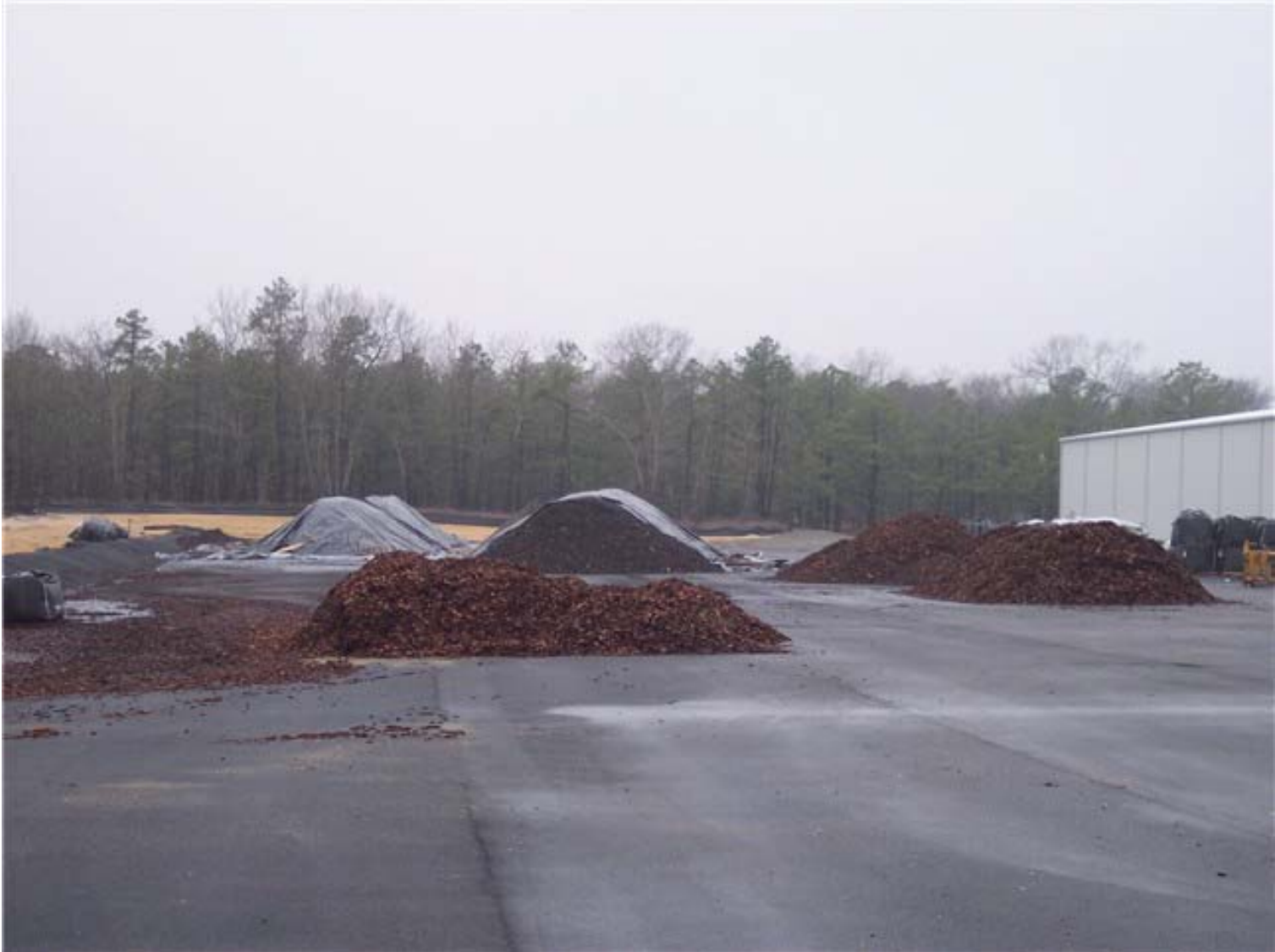
The bio-filters are filled with a media that contains wood chips, soil from the site and carbon.
