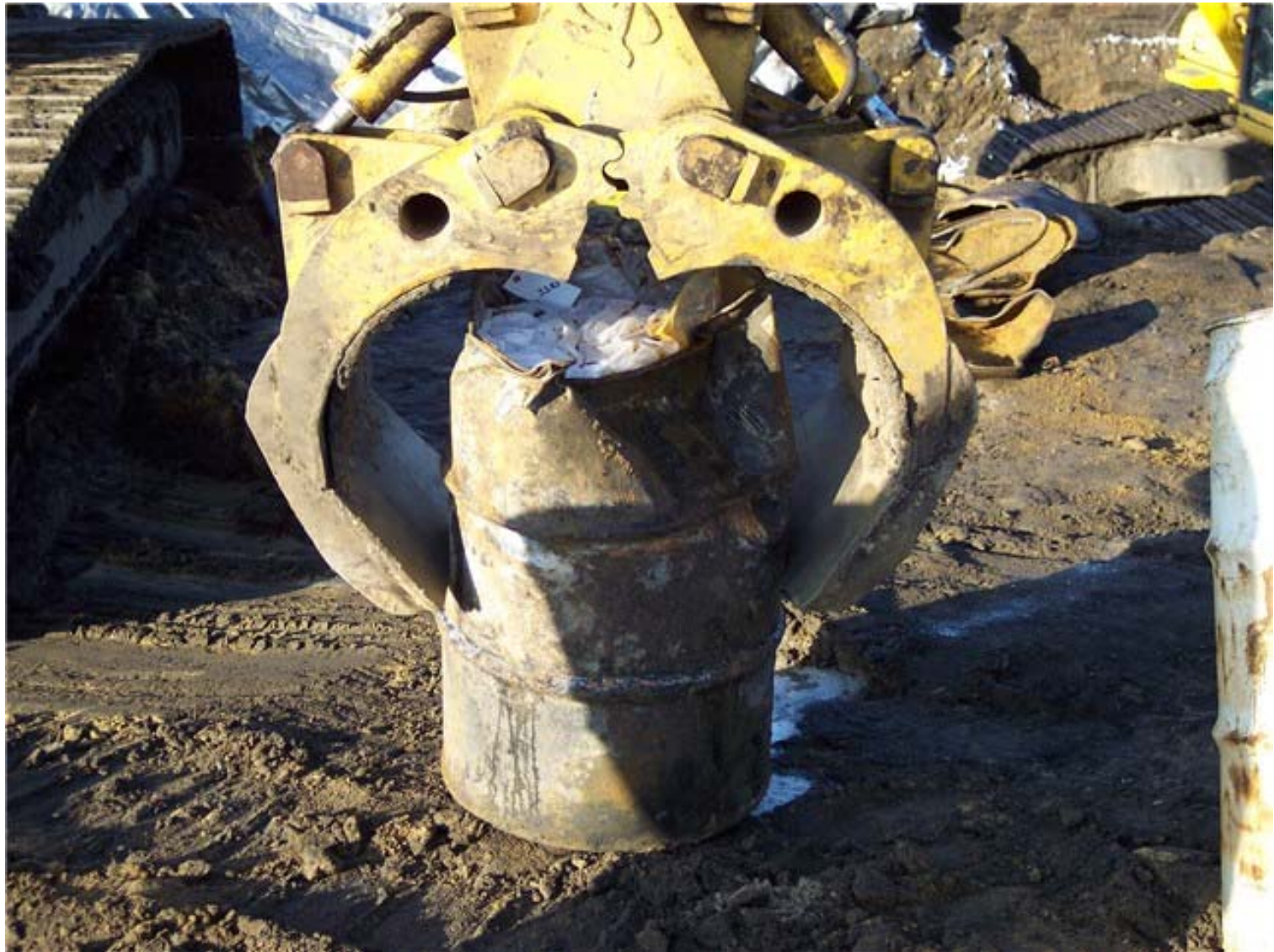
Drums are removed from the excavation using a piece of heavy equipment fitted with a grapple.
