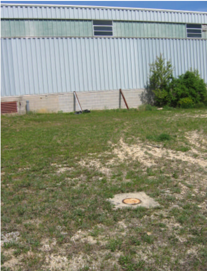
Soil Venting/Sparging System - Well
