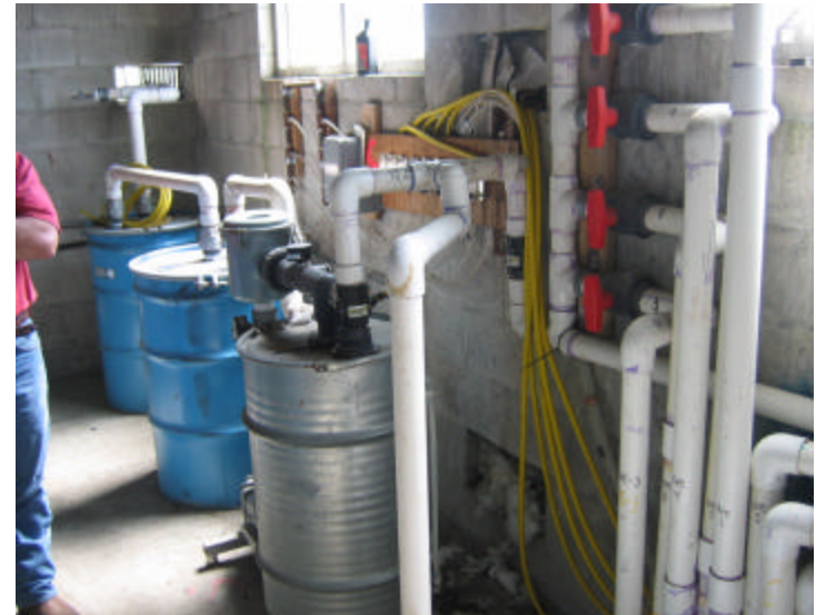
Soil Venting/Sparging System - Treatment Units & Piping (Housed in Area G)
