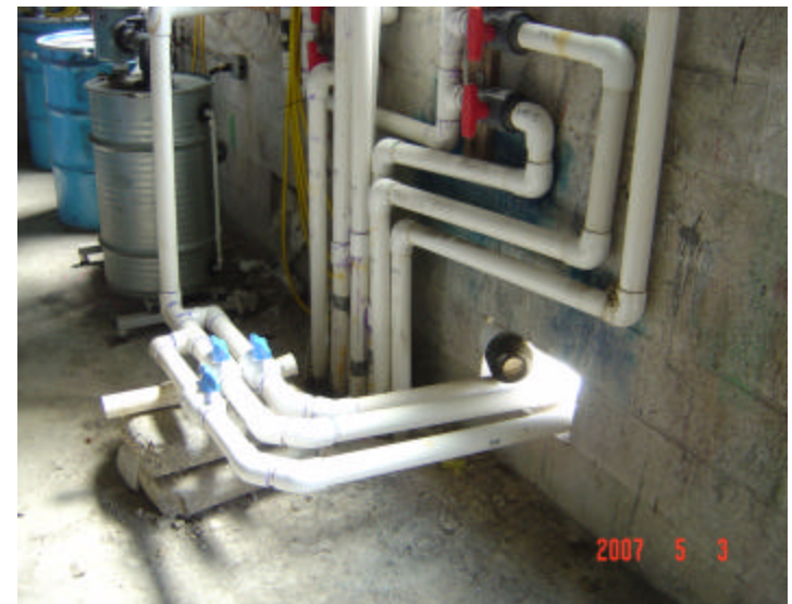
Soil Venting/Sparging System - Treatment Units & Piping (House in Area G)
