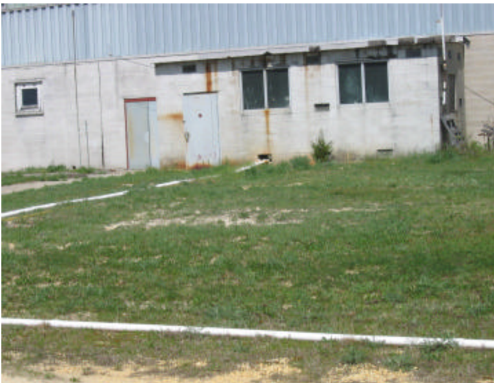
Area P-2 (Underground Concrete Vault #2) & Area G (Former Empty Solvent Drum Storage Area), View to the North
