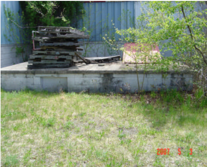
Area L (Non-Contact Cooling Water Recycling Tank), View to the South
