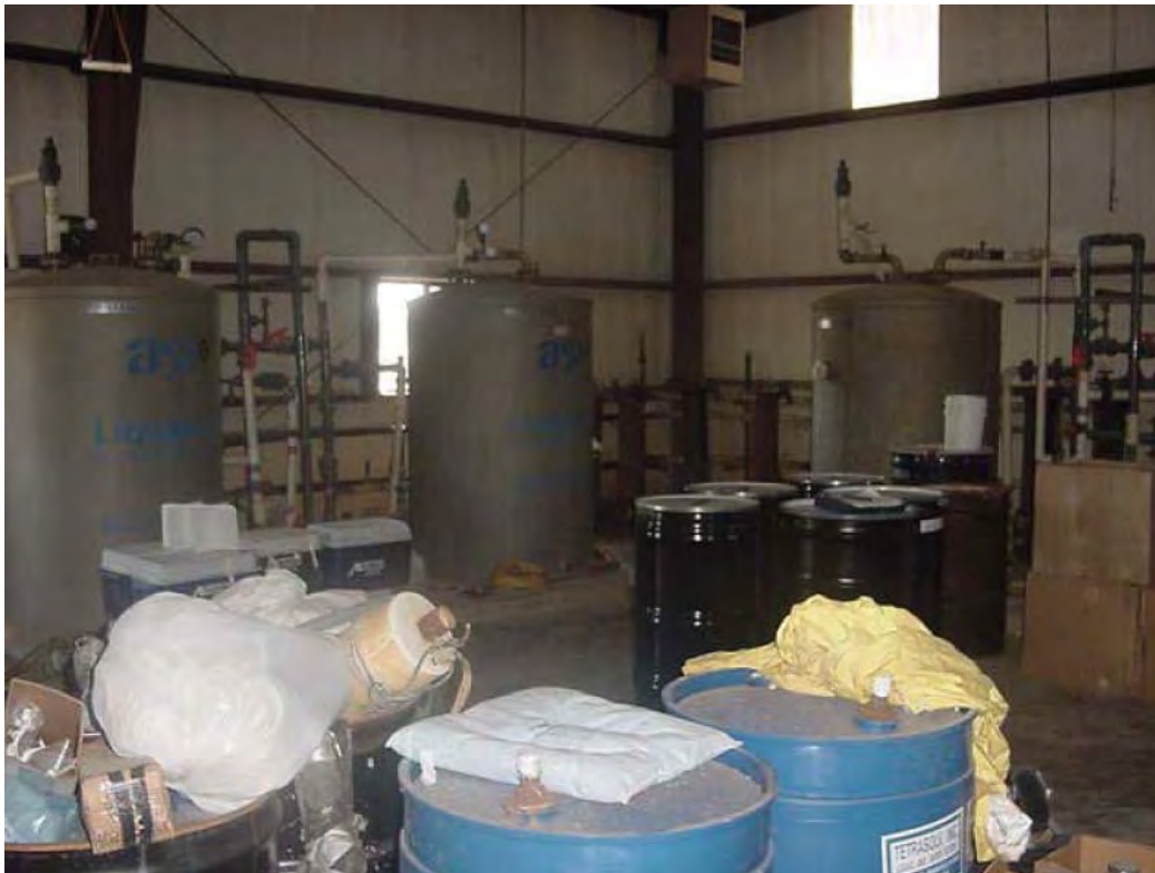
Photo 6: Activated carbon canisters and fabric filters on south side of WWTP
