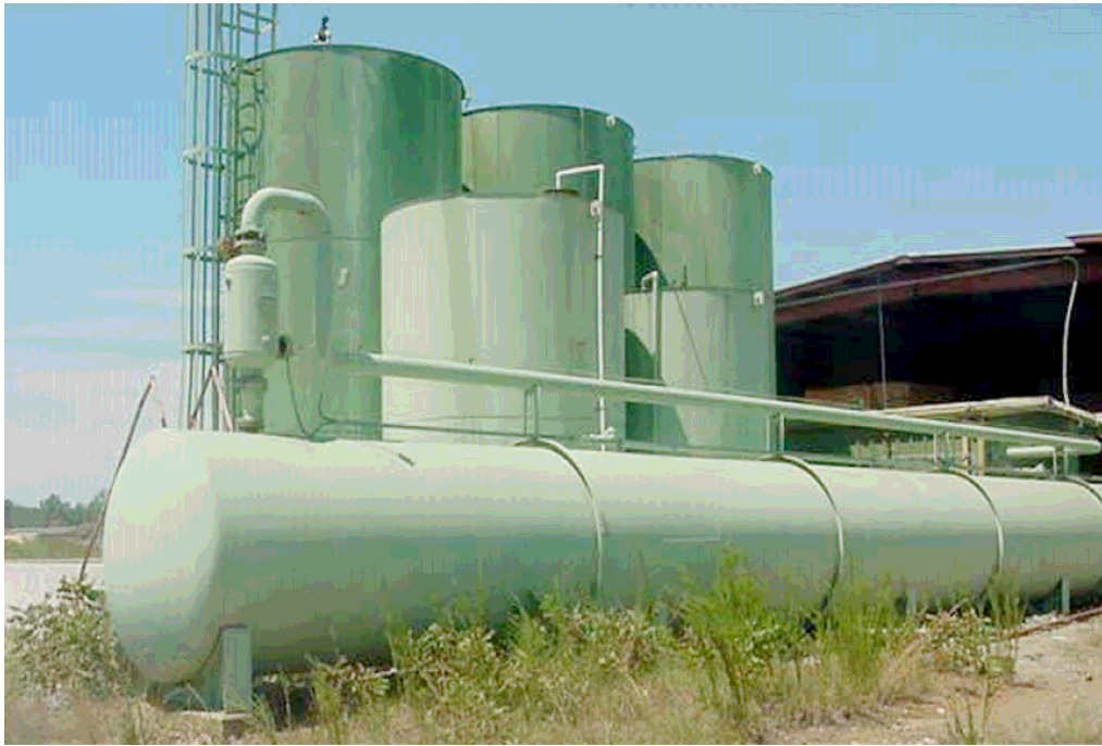
Photo 3: Chromated Copper Arsenate (CCA) treatment cylinder and storage tanks
