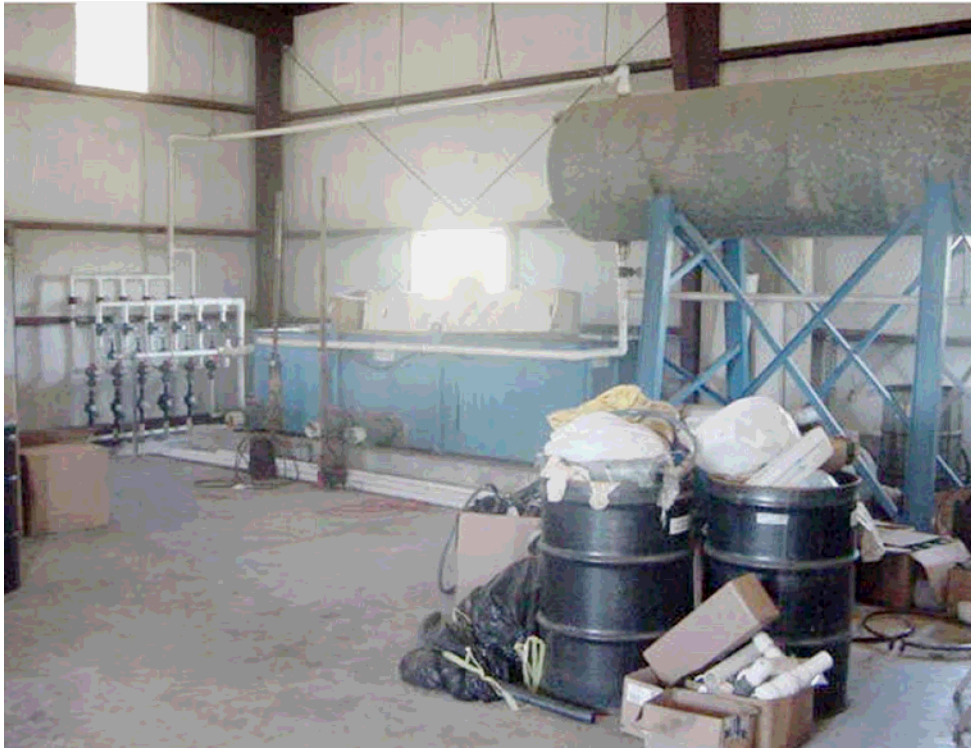
Photo 1: Oil-Water separator within wastewater treatment plant (WWTP)
