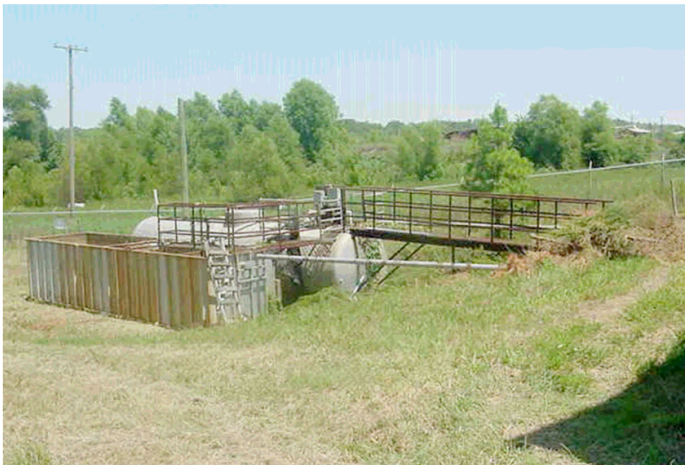
Photo 2: Storage and Overflow tanks north of (WWTP)
