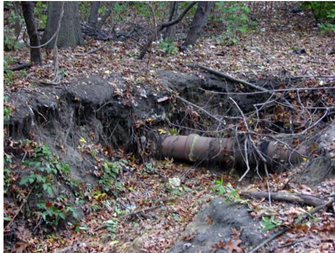
Figure 3 - - Gully erosion, pipe exposed
