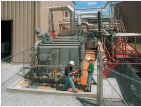
Thermal oxidizer on its concrete pad outside the treatment building.
