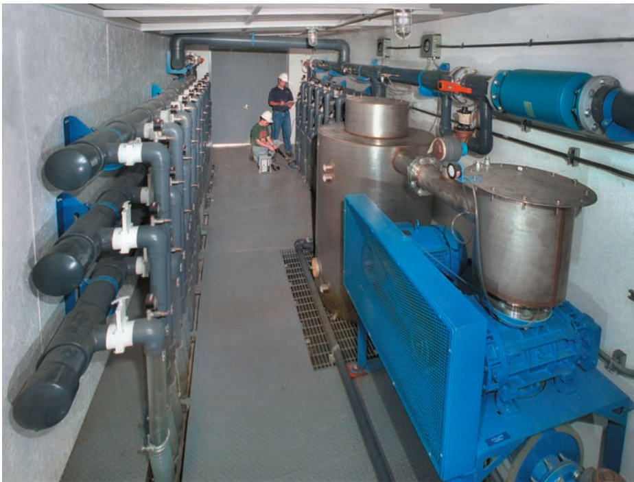
View of the inside of the SBPA blower shed. Two MWH engineers are shown taking readings from one of the sampling ports on the header system.
