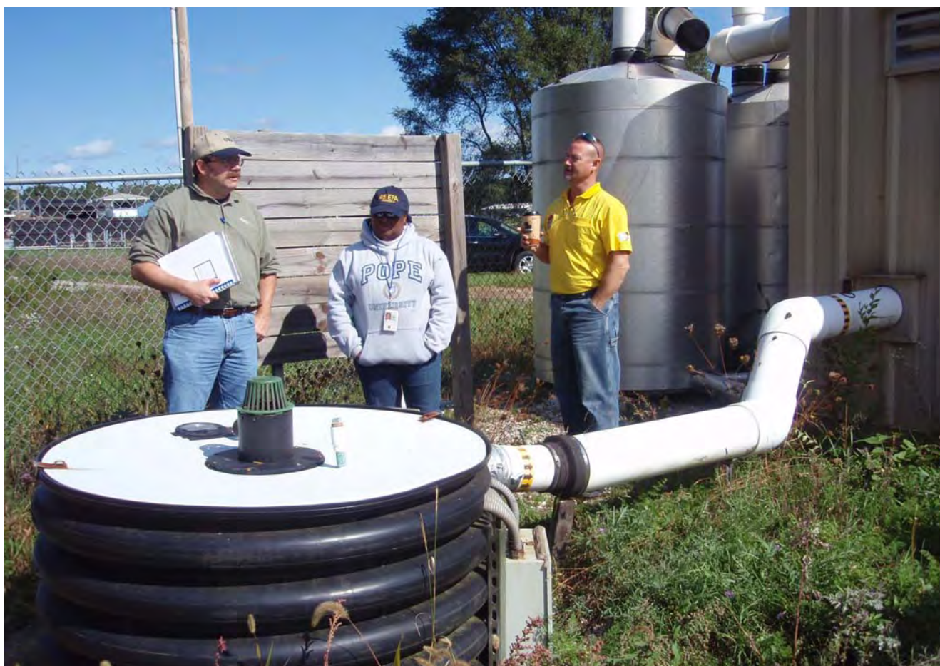
Drag Strip Area Groundwater Recirculation Well
