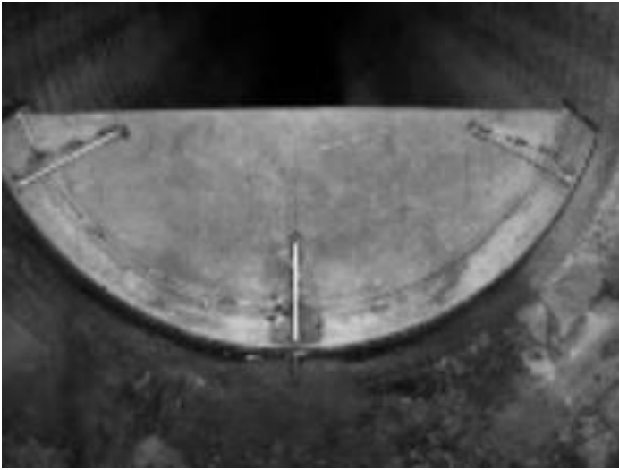
Top photo shows a weir sitting in the Ten-Mile Drain. The weirs act like small dams collecting polluted oil and sediment before the contaminants can move into the canals.
