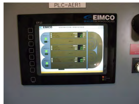
New SCADA control interface
