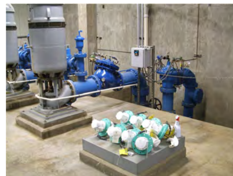
New high service pumps
