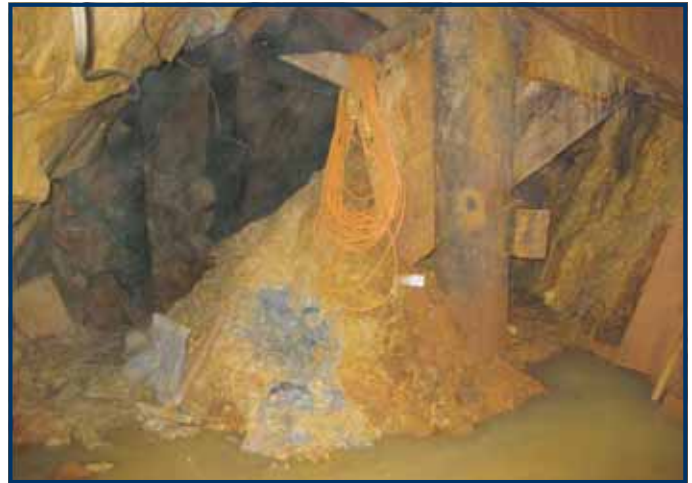
Figure 6—Muck Pile and Water in Level 3 Tunnel
