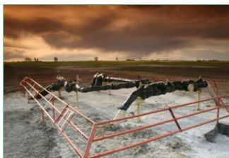
Landfill gas energy project in Alberta, Canada
