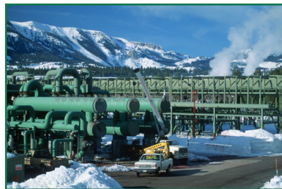
A geothermal power plant in Mammoth Lakes, CA
