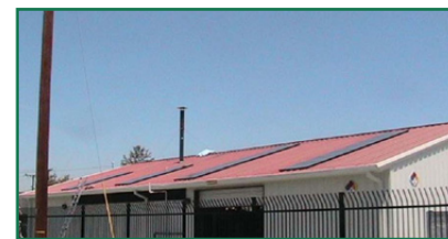
PV roof panels in Pemaco, CA
