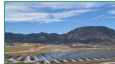
A PV array at Fort Carson, CO
