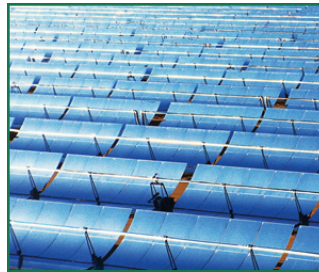
A CSP trough system
