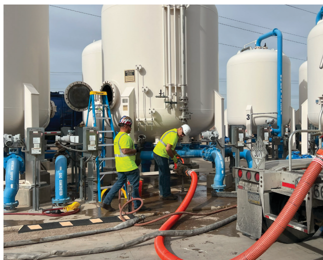
Changeout in progress for a granular activated carbon (GAC) treatment system for PFAS. GAC is a proven technology for removing PFAS from drinking water and is already in use in many communities.
