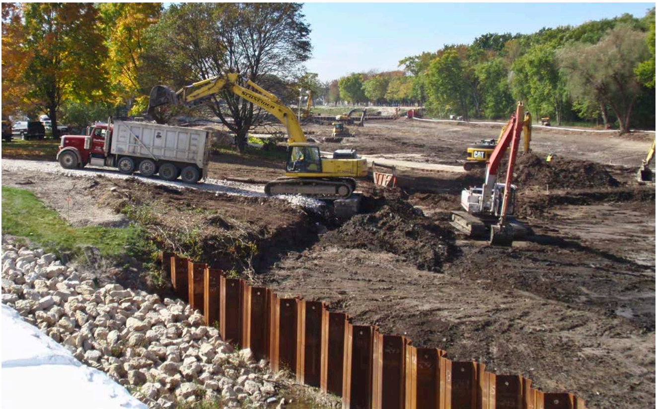
Contaminated sediments being excavated from the project area and loaded onto trucks.
