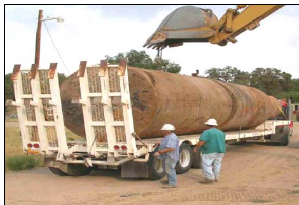
The Jicarilla Apache Environmental Protection Office overseeing UST removals on the Jicarilla Apache Nation
