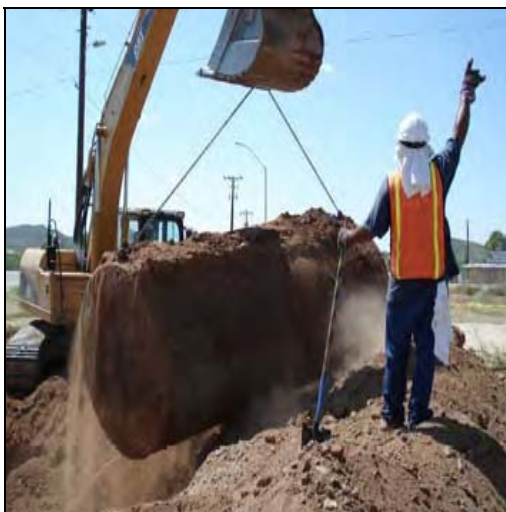
An UST is removed during a site assessment on the Tohono O'Odham Nation
