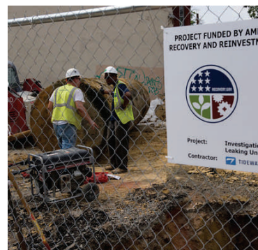
LUST Recovery Act money is helping clean up this site in Washington, D.C.
